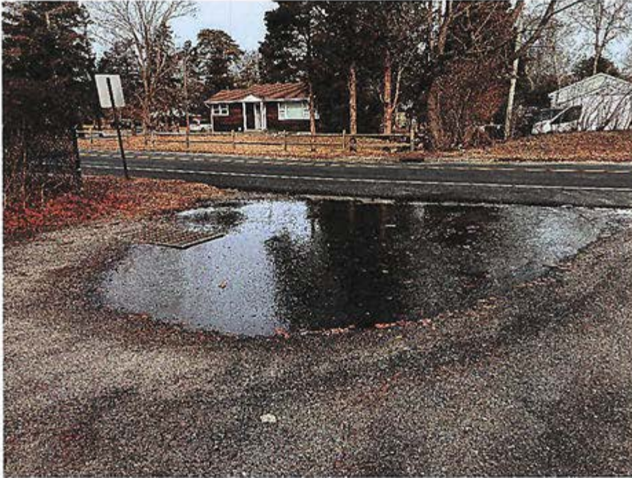
Area of existing ponding and fail drainage.
