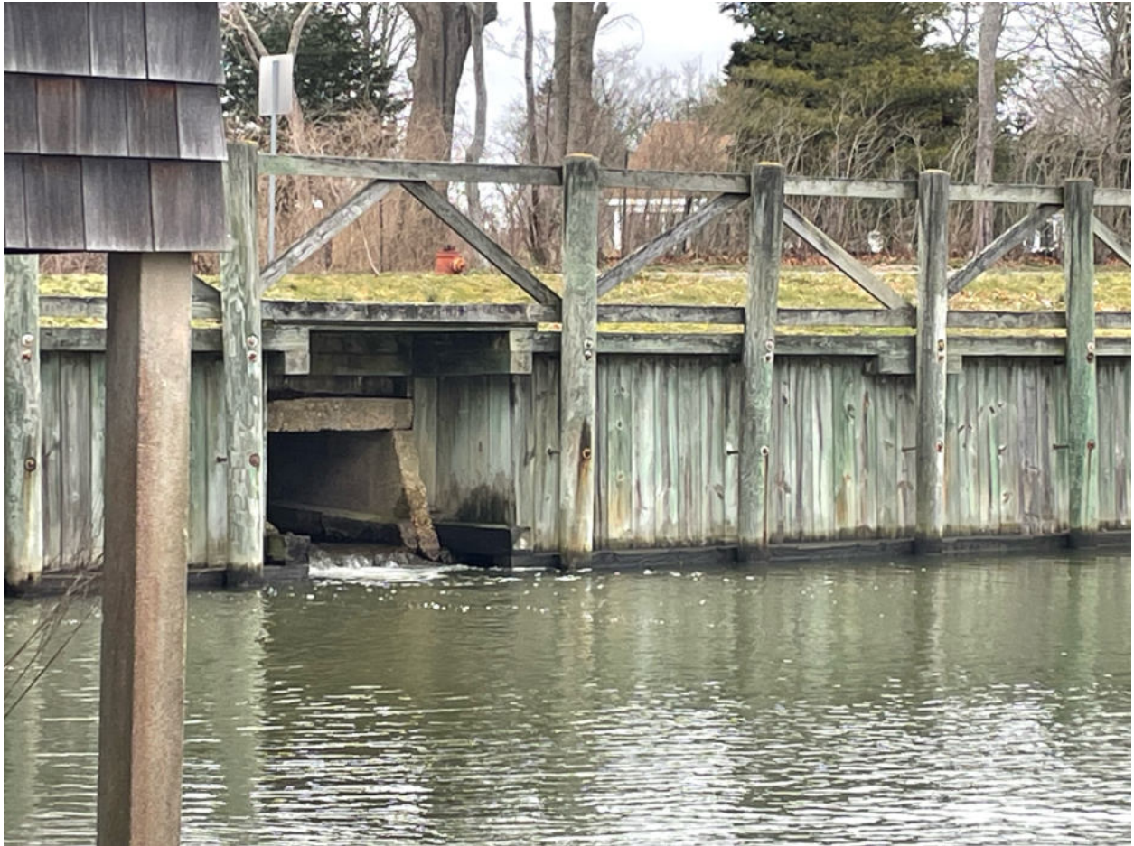
Photo 1. Bulkhead and existing culvert. Fish passage will be built within the culvert area.
