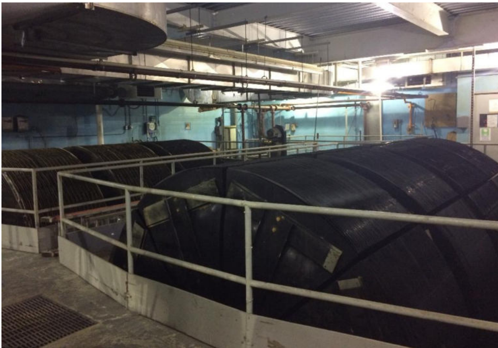
Figure 3-4 Rotating Biological Contactor SH STP
