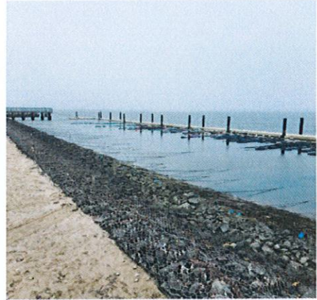
c. A new nursery net system will be installed at Tiana Bayside
