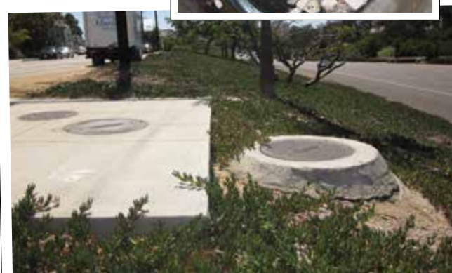
A CDS was installed to pretreat for a bioswale in Newport Beach, CA
