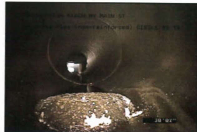
Photo: 6_1_2_13092016_104043_B.JPG, VCR No.: DVD01 TV-91 28FT, Deposits Settled Compacted, 5 %of cross sectional area, from 05 to 07 o'clock, , within 8 inches of joint: YES
